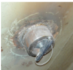
Permanently fitted Tube Socket. When build up occurs sealing plug is taken out and tube inserted through socket.
